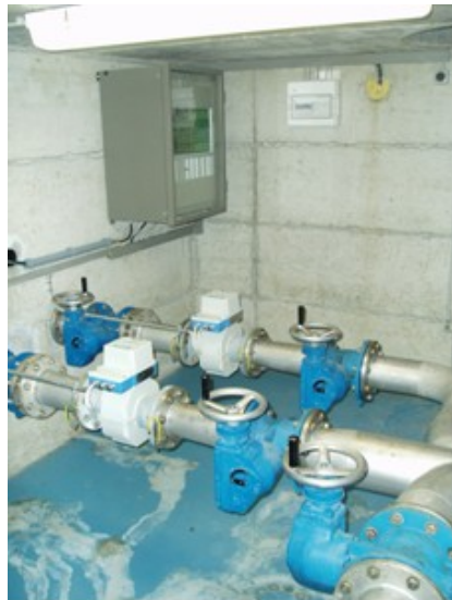
Station de pompage Montasson
